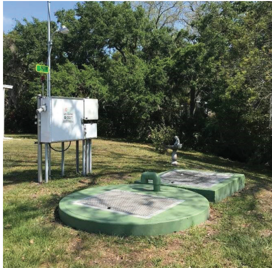
Figure 6: Overview of Lift Station No. 521 (Colony Cove 4)
