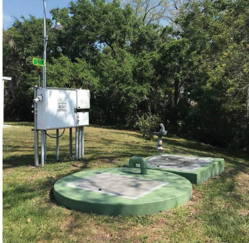
Figure 8: Overview of Lift Station No. 521 (Colony Cove 5)
