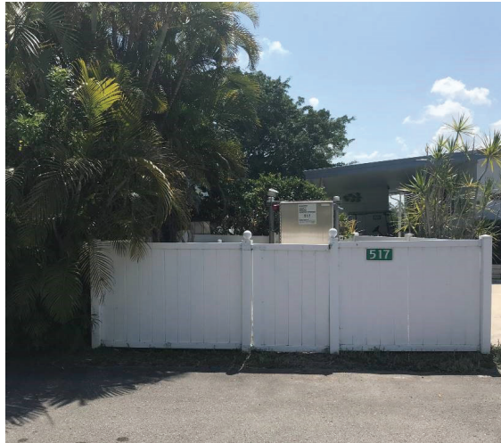
Figure 2: Overview of Lift Station No. 517 (Colony Cove 1)
