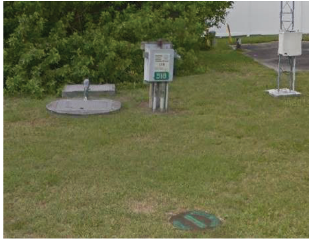
Figure 3: Overview of Lift Station No. 518 (Colony Cove 2)
