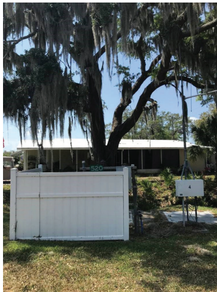
Figure 5: Overview of Lift Station No. 520 (Colony Cove 4)
