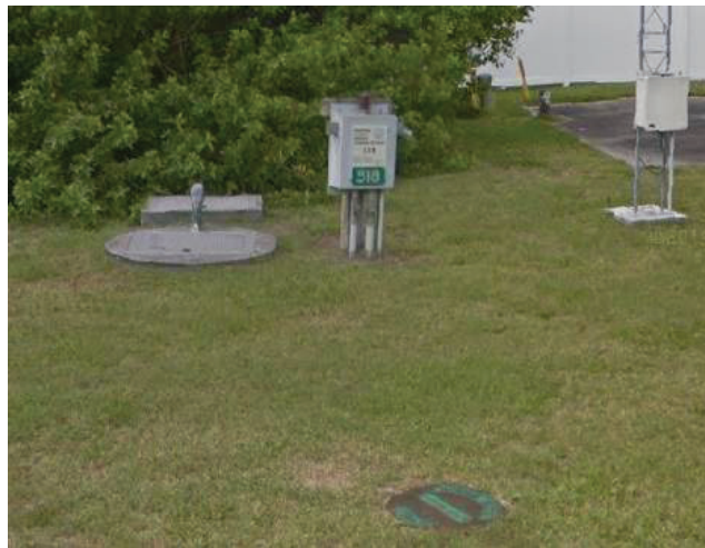
Figure 5: Overview of Lift Station No. 518 (Colony Cove 2)
