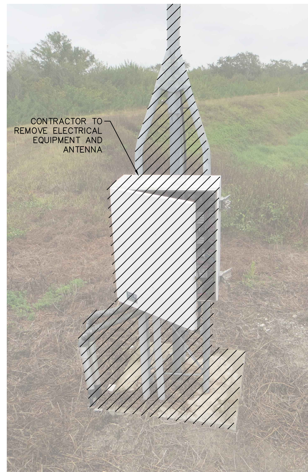
EX. EAST LAKE ELECTRICAL EQUIPMENT
