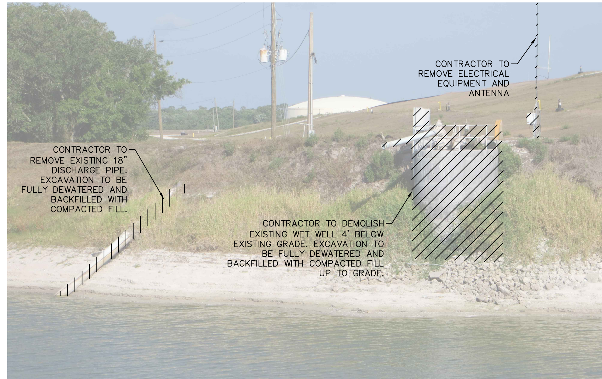
EX. EAST LAKE PUMP STATION
