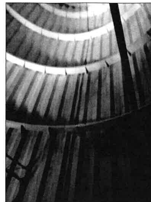
EXISTING SCADA RADIO ANTENNA CABLES
