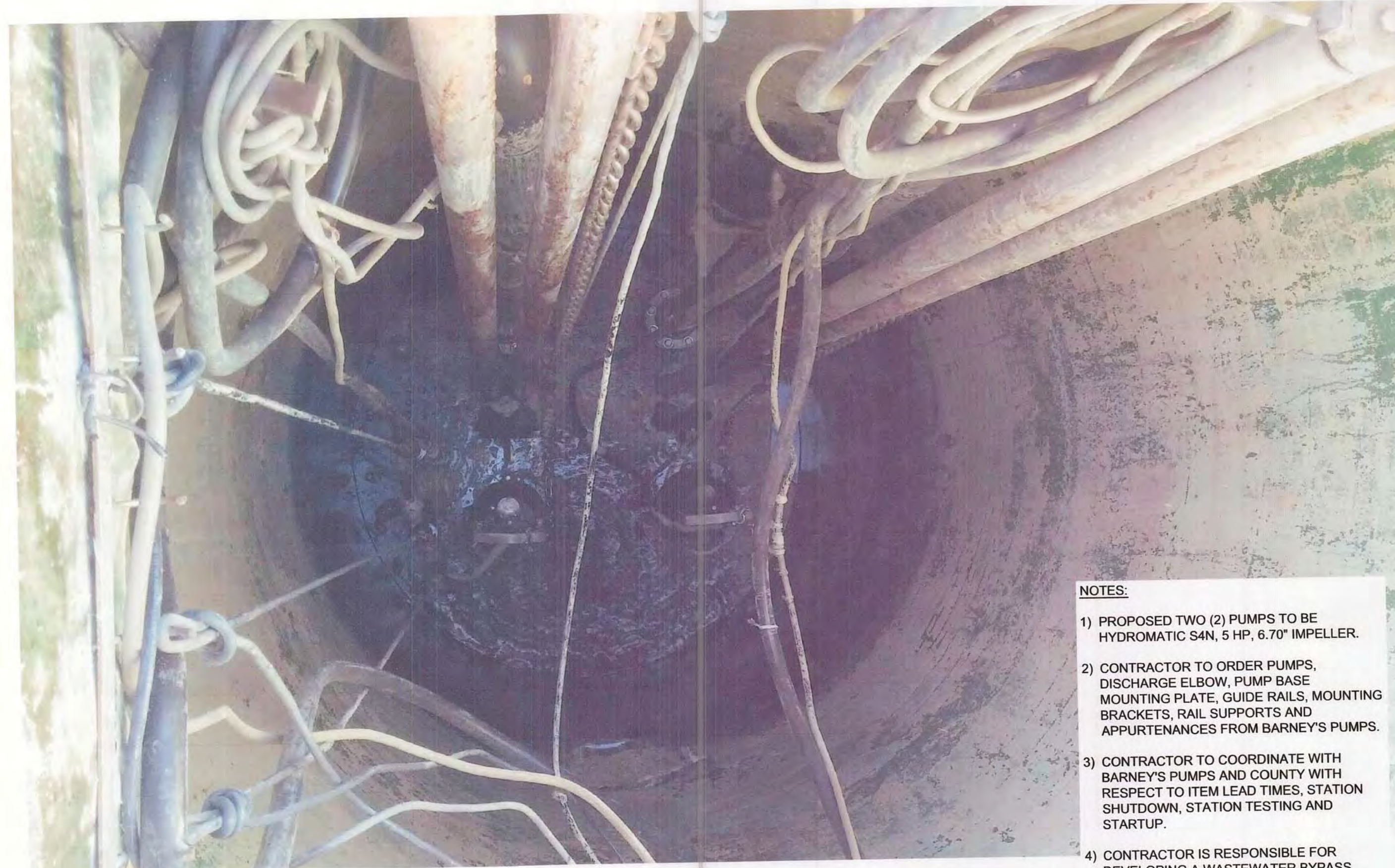
REPLACE EXISTING PUMPS, DISCHARGE ELBOWS, GUIDE RAILS AND APPURTENANCES AND INSTALL PUMP BASE MOUNTING PLATE
