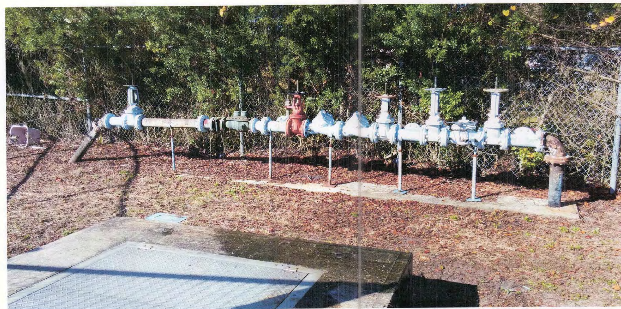
WATER MAIN/BACKFLOW PREVENTER ASSEMBLY ABOVE GRADE (REPAINT)
