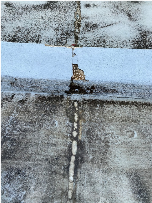
Condition L – Location: slab expansion joint material deterioration.
