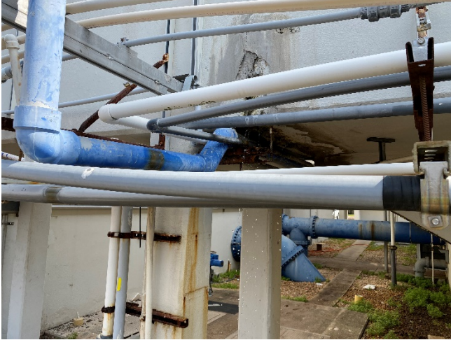
Condition K – Location: leak through expansion joint.
