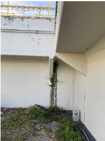
Condition J – Location: expansion joint material deterioration.
