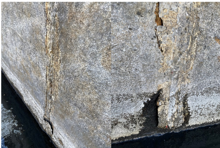
Condition D – Location: damage of expansion joints surrounding concrete.
