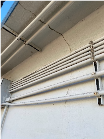
Condition I – Location: crack formation on the outside face of perimeter wall.
