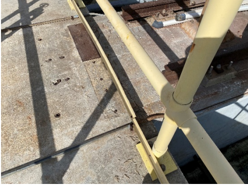
Condition H – Location: cracks on walkway slab.
