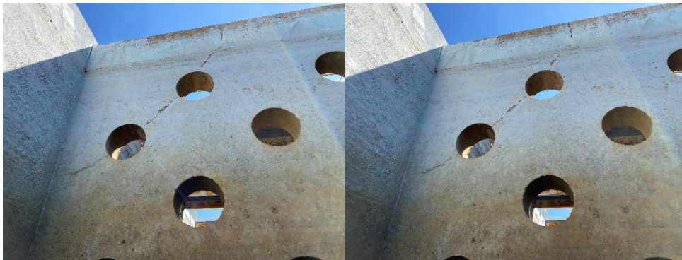
Condition C – Location: formation of diagonal cracks on baffle walls.
