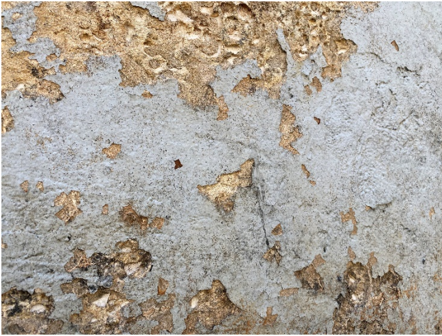
Condition F – Location: coating decay at walls.
