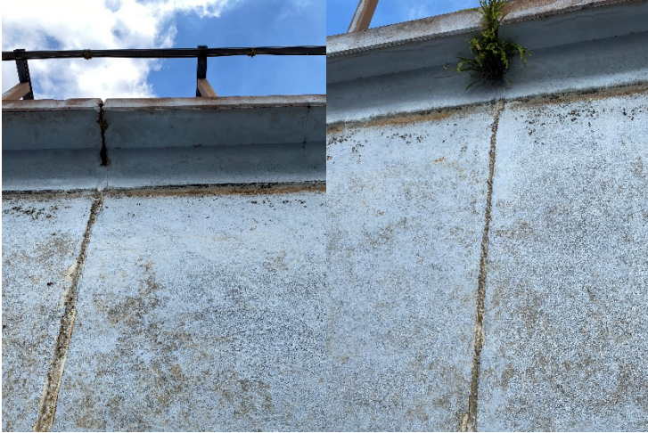
Condition E – Location: wall expansion joint material deterioration.
