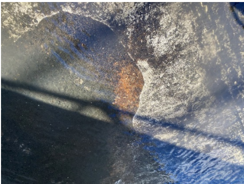
Condition G – Location: slab appears to show concrete degradation over South-West corner of South Train.
