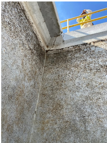
Condition A – Location: cracks on walkway slab.
