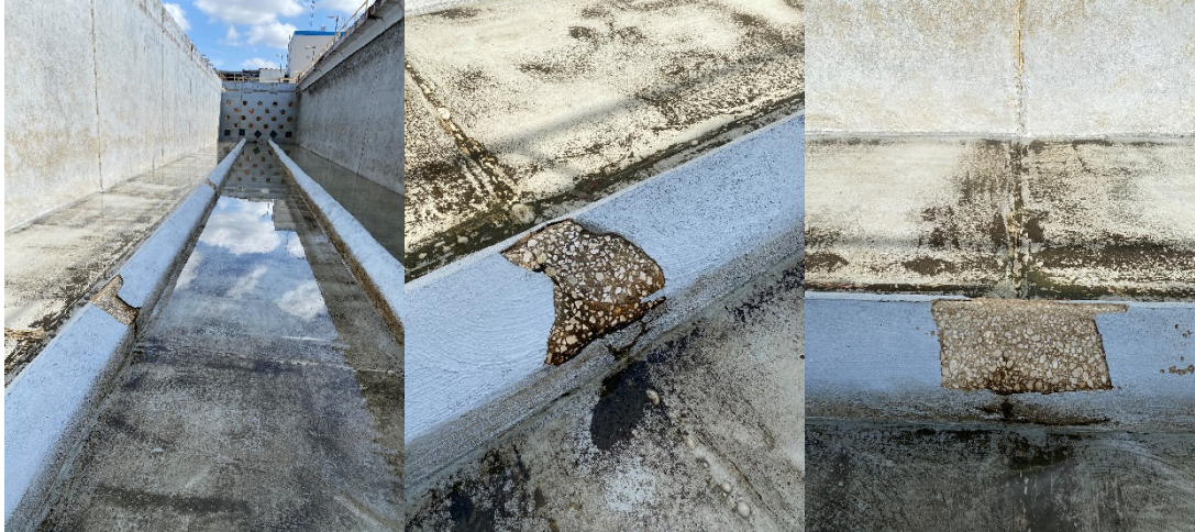
Condition B – Location: spalling of mortar (wearing surface) at curbs.
