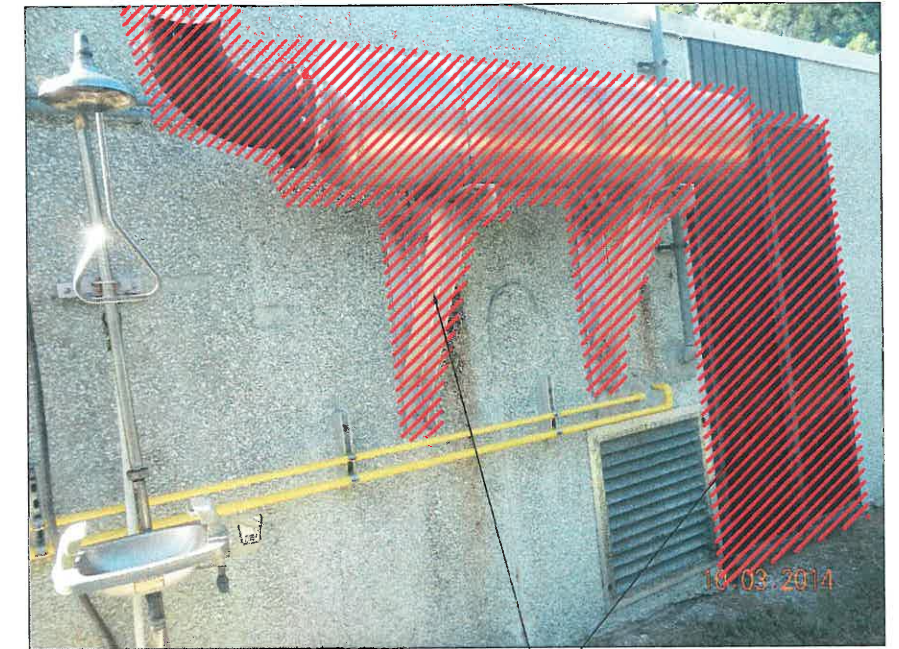
PHOTOGRAPH #1 - TYPICAL VIEW OF EXTERIOR OF BUILDING SHOWING LOUVER AND EXHAUST MUFFLER.
