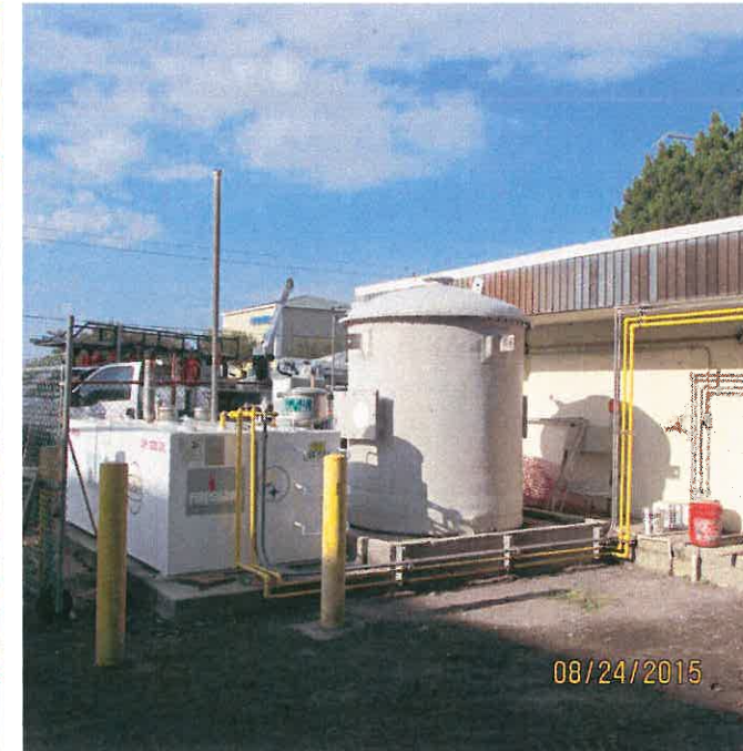
PROPOSED GENERATOR LOCATION (FACING SOUTHWEST)
