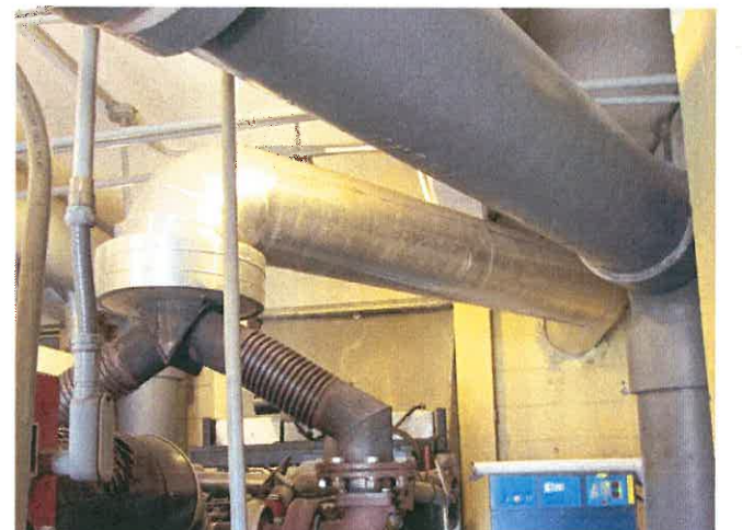
EXISTING GENERATOR EXHAUST DUCT (TO BE REMOVED)
