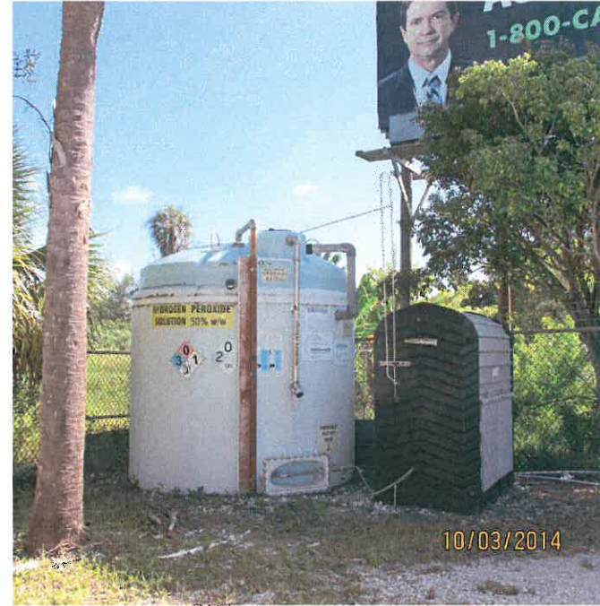
EXISTING CHEMICAL TANK W/ ACCESSORY (FACING NORTHEAST)
