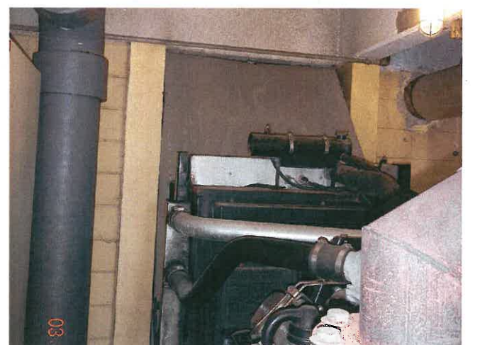
EXISTING GENERATOR RADIATOR AND DUCT (TO BE REMOVED)
