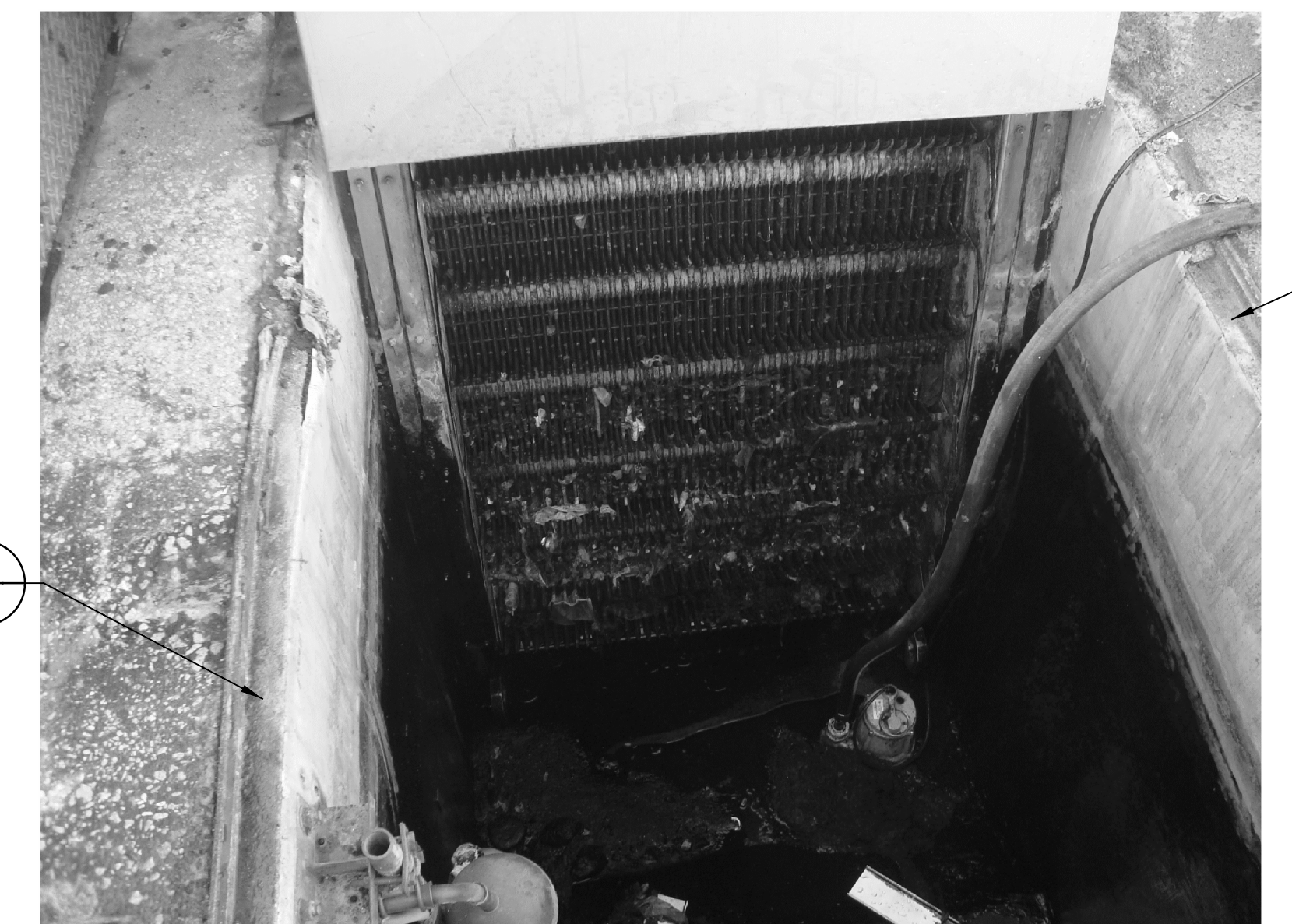
D REPAIR SOFTENED CONCRETE AT REBATE
