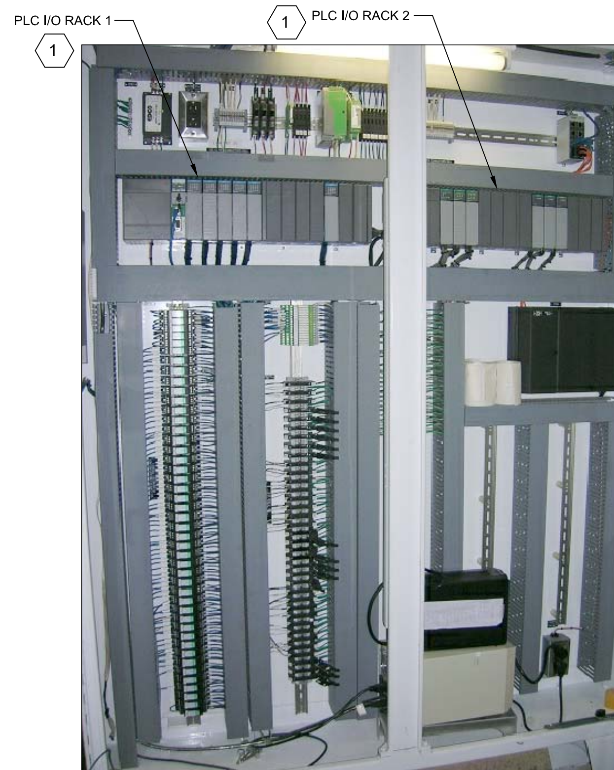
EXISTING HEADWORKS PLC PANEL - INTERIOR NOT TO SCALE
