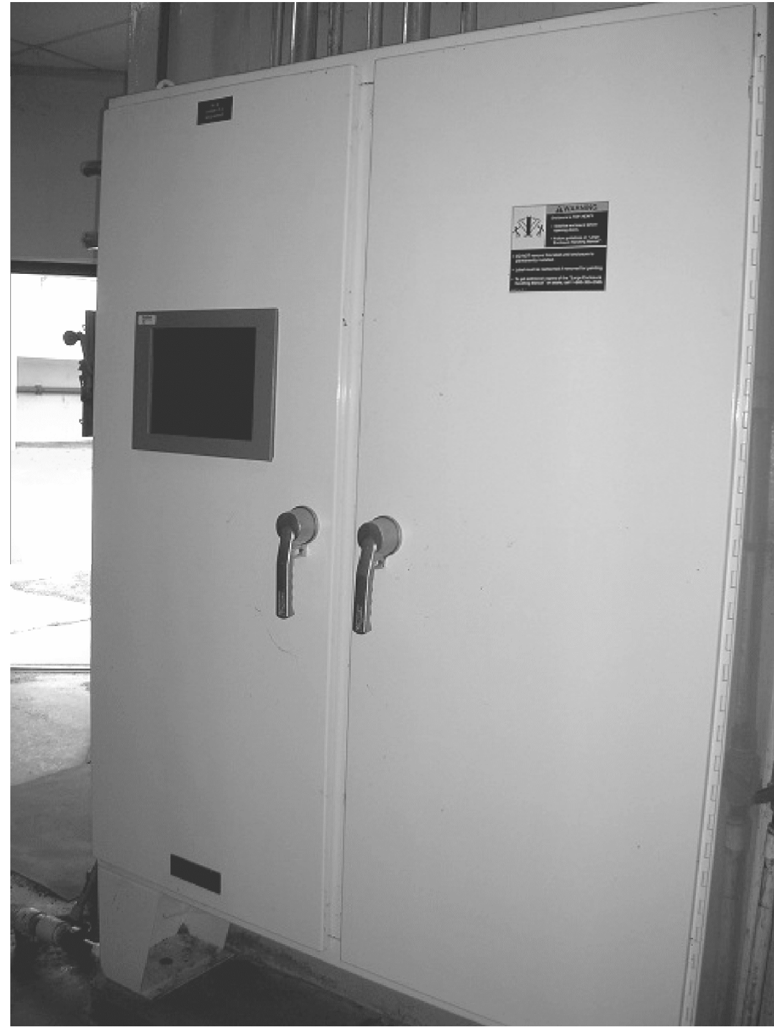
EXISTING HEADWORKS PLC PANEL NOT TO SCALE
