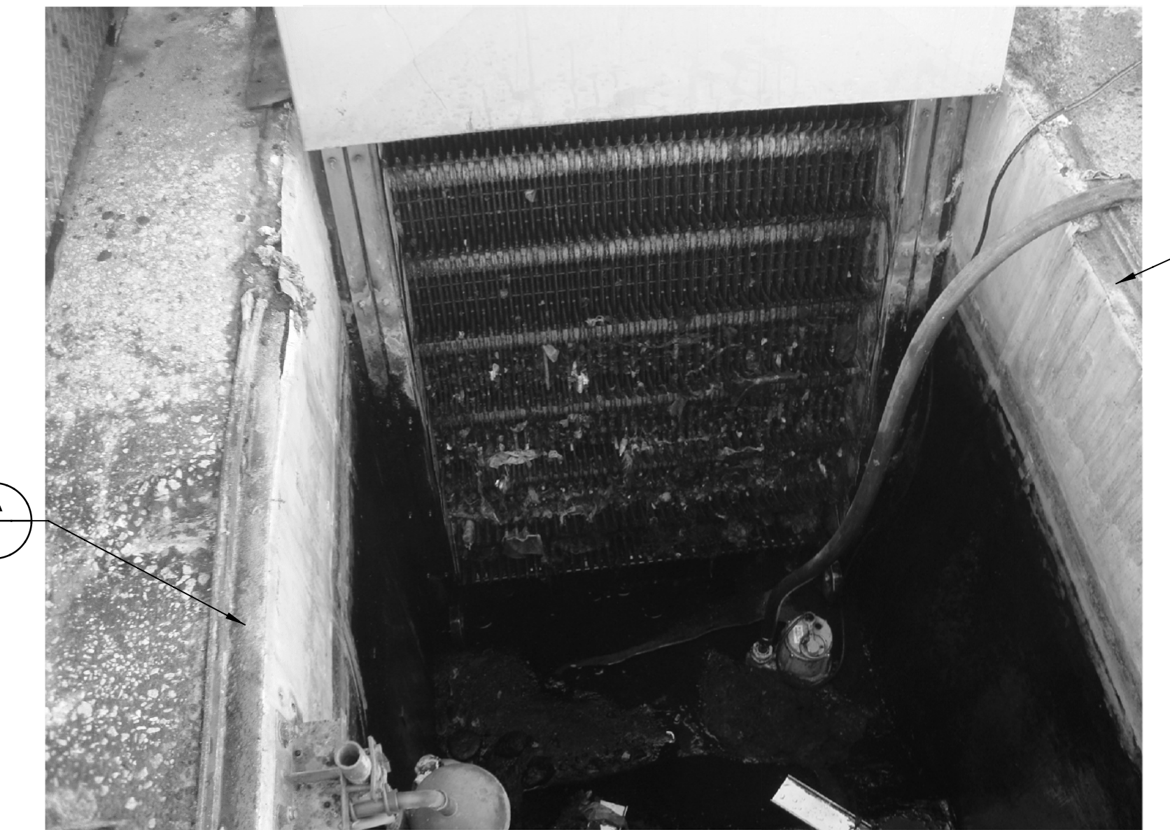
D REPAIR SOFTENED CONCRETE AT REBATE
