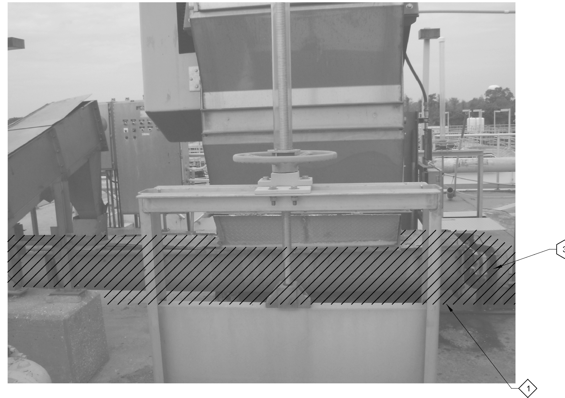
2 CONVEYOR NO.1 DETAIL FILE: SCREW CONVEYOR 1.JPG
