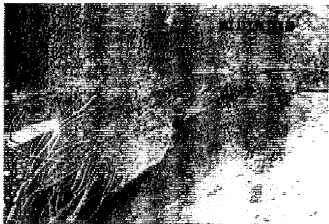
I - Infiltration @ 154.5 ft. water
