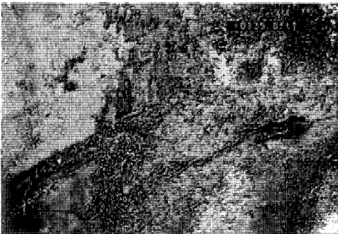
I - Infiltration @ 135.8 ft. water
