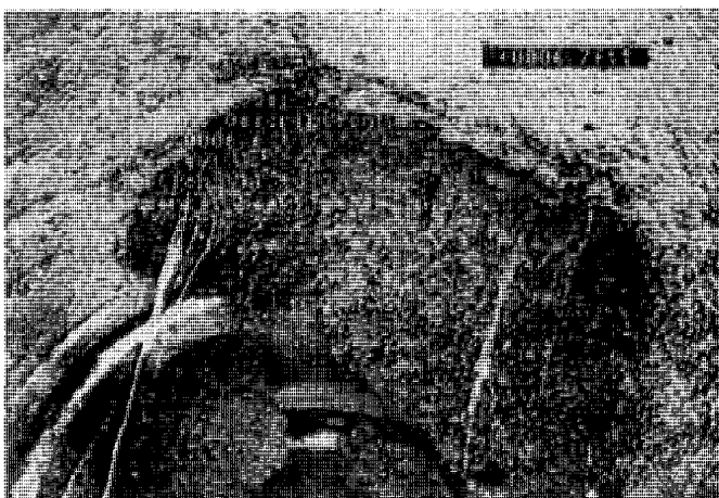
R - Roots @ 6.6 ft. heavy water infil
