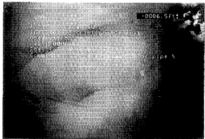
GO - General Observation @ 6.5 ft. concrete on bottom of pipe \
