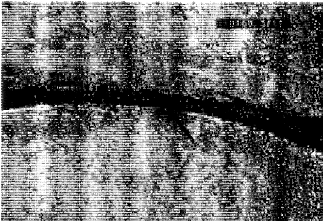
R - Roots @ 160.3 ft. light in joint
