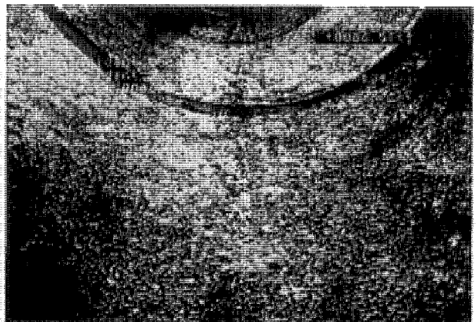
SD - Surface Damage @ 84.5 ft. aggregate visible
