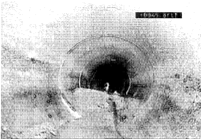
ACB - Access point CB @ 45.8 ft.
