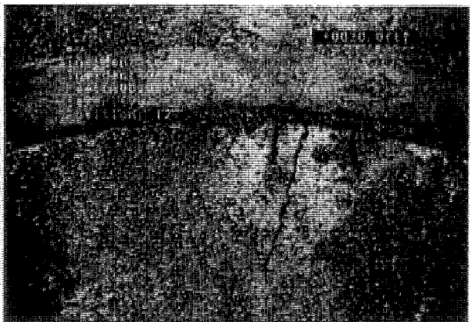
C - Crack @ 30.0 ft. surface crack
