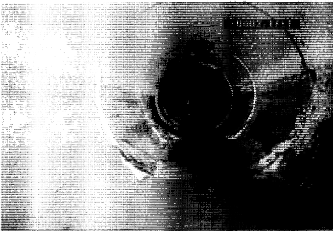
ACB - Access point CB @ 0.0 ft.
