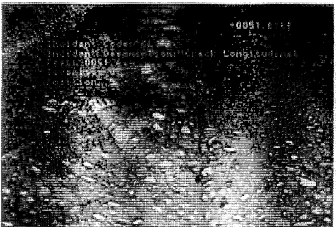
CL - Crack Longitudinal @ 51.6 ft. surface spalding & crack
