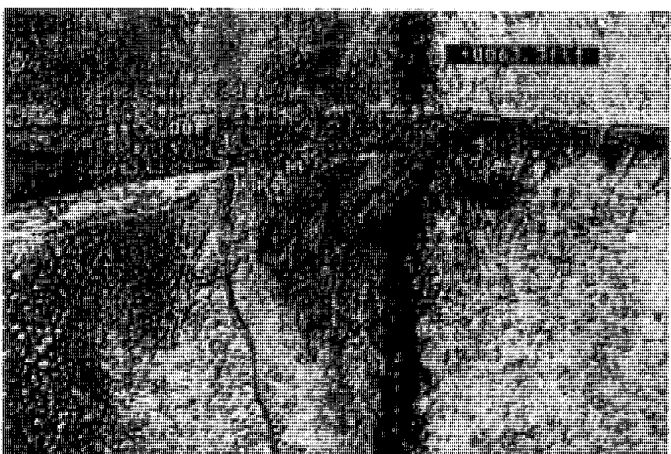
R - Roots @ 63.3 ft. light from joint
