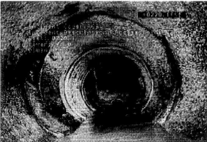
ACB - Access point CB @ 220.1 ft.
