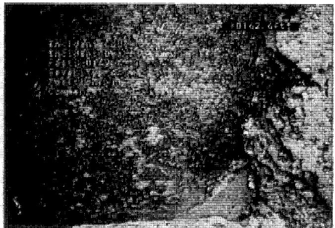
H - Hole @ 142.4 ft. void visible
