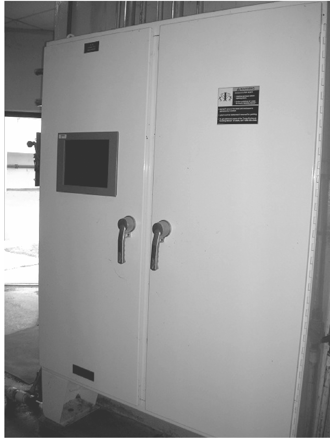
EXISTING HEADWORKS PLC PANEL NOT TO SCALE
