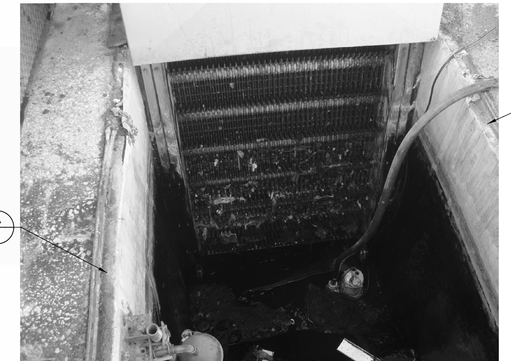
D REPAIR SOFTENED CONCRETE AT REBATE
