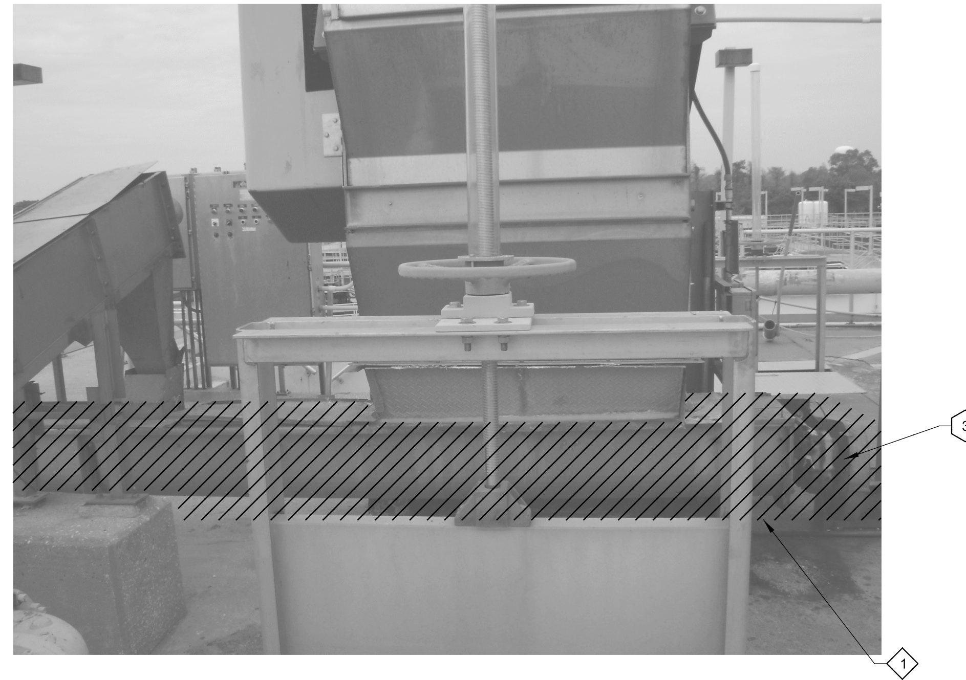
2 CONVEYOR NO.1 DETAIL FILE: SCREW CONVEYOR 1.JPG
