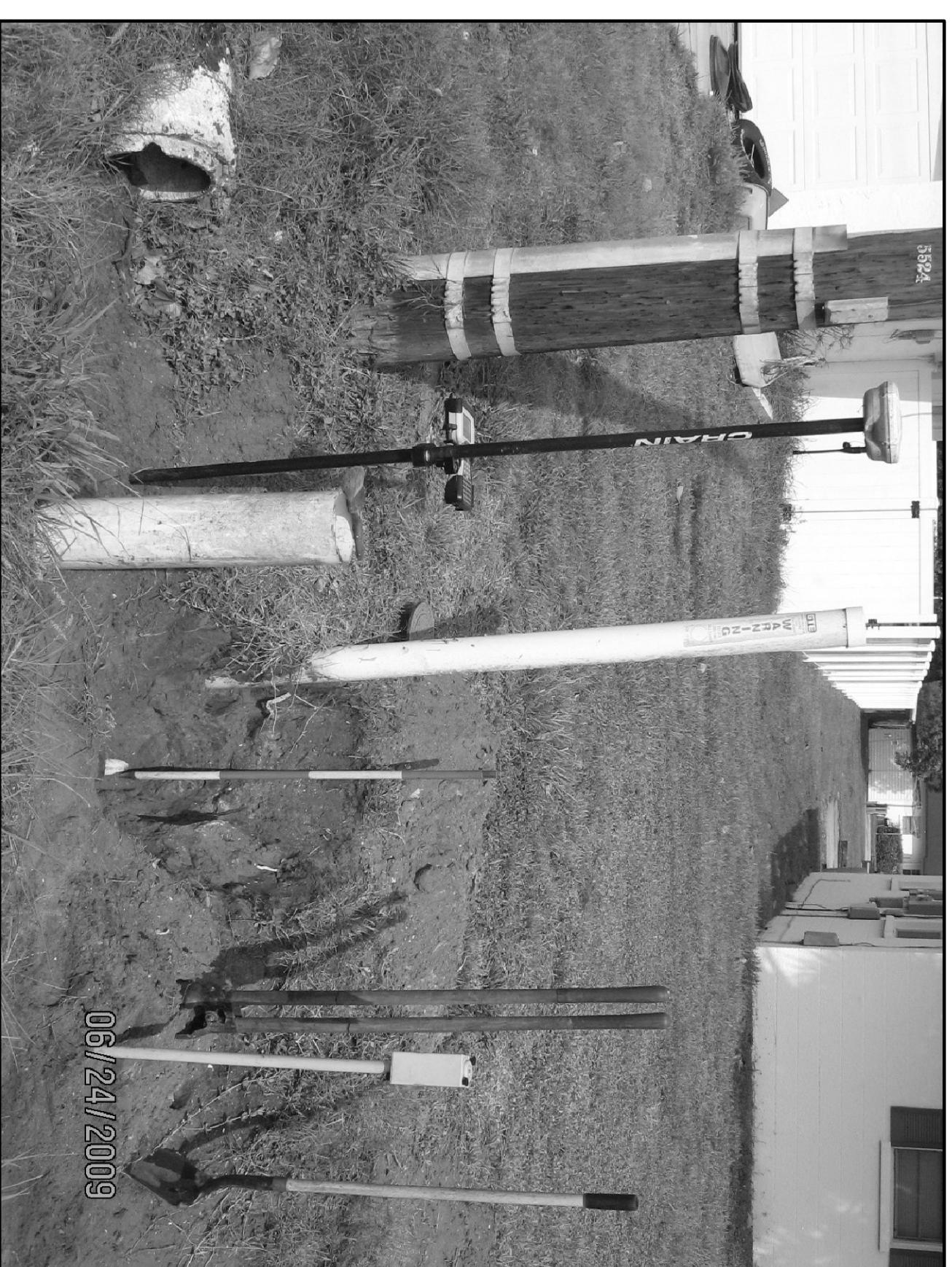
EXCAVATION - NORTH VALVE LOCATION ON 25th ST W AT SOUTH PROP LINE OF 5518 25TH ST W
