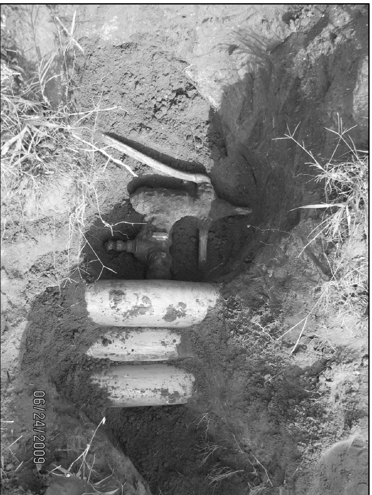
EXCAVATION - NORTH VALVE LOCATION ON 25th ST W AT SOUTH PROP LINE OF 5518 25TH ST W
