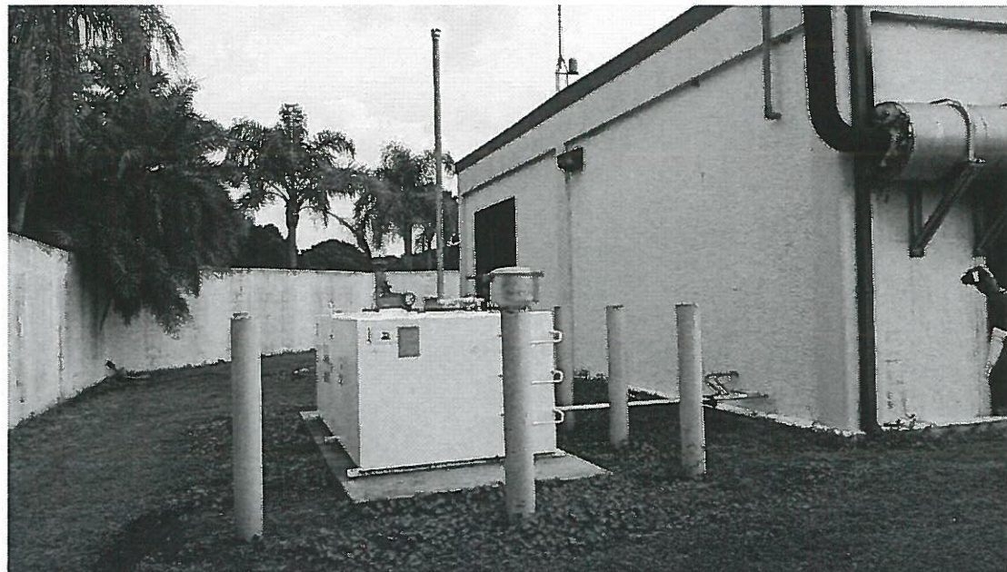
EXISTING DIESEL TANK - TO BE REMOVED (FACING EAST)
